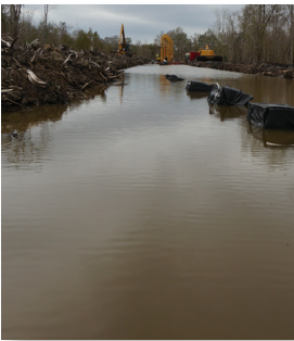
Pipeline is submerged 2 m (6 ft) below the swamp, crossing environmentally sensitive wetlands
